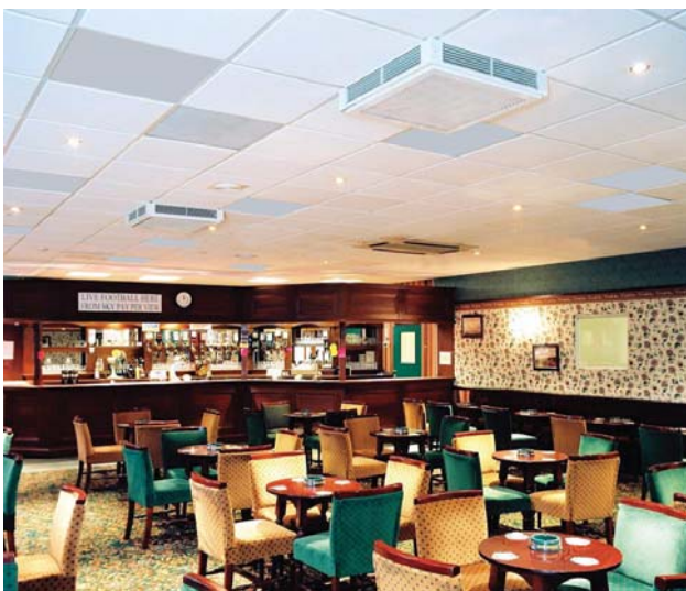
PA120 Concealed into a ceiling.
